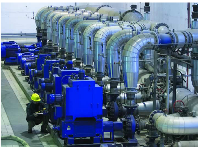
© HERA. District Heating Pumps.
